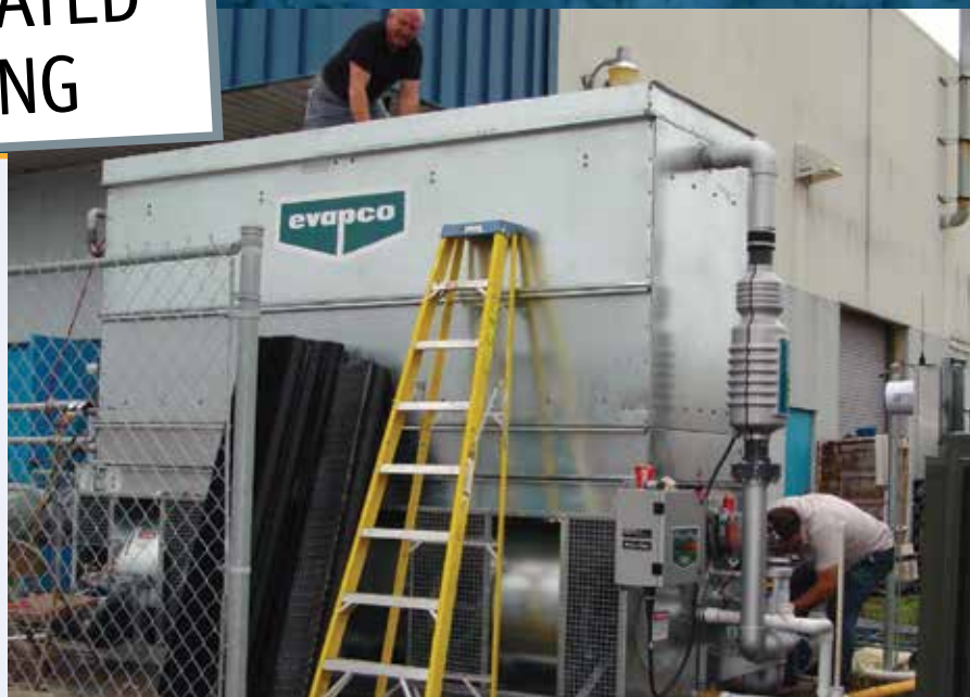
Condensers require regular maintenance before, throughout, and after the skating season.
