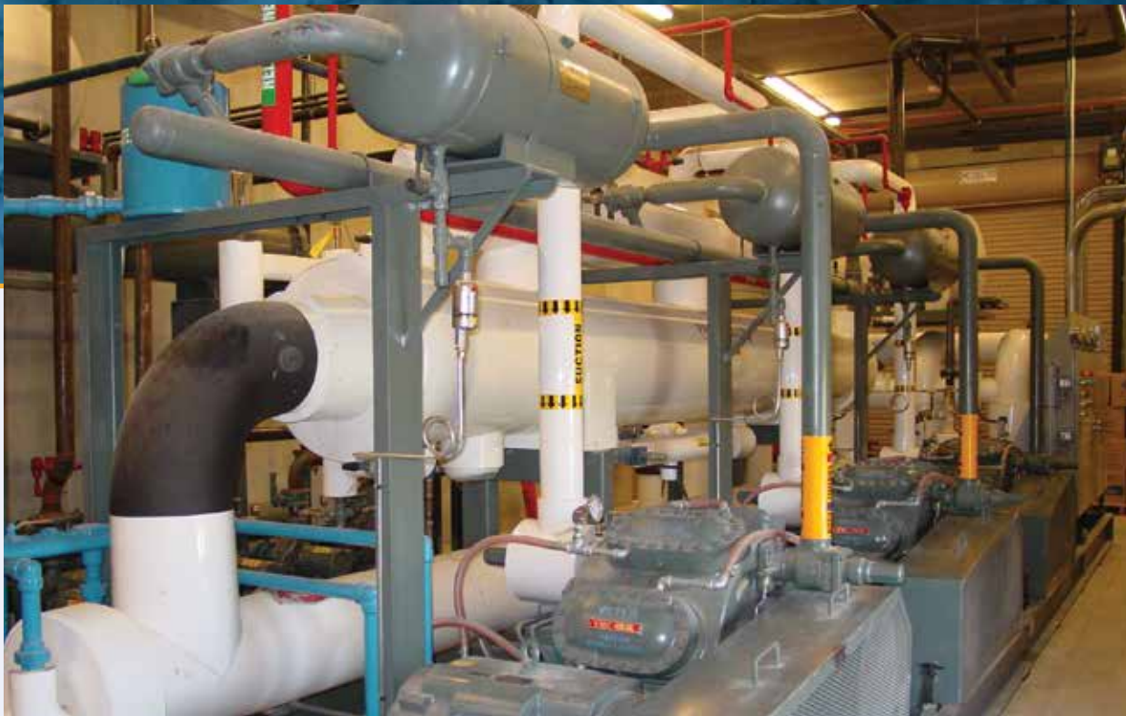
Refrigeration skid with reciprocating compressors.
